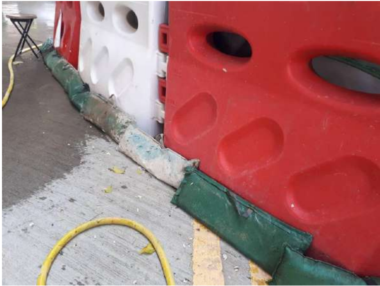
Figure A6: Sandbags were provided along the site boundary for site in Zone B2
